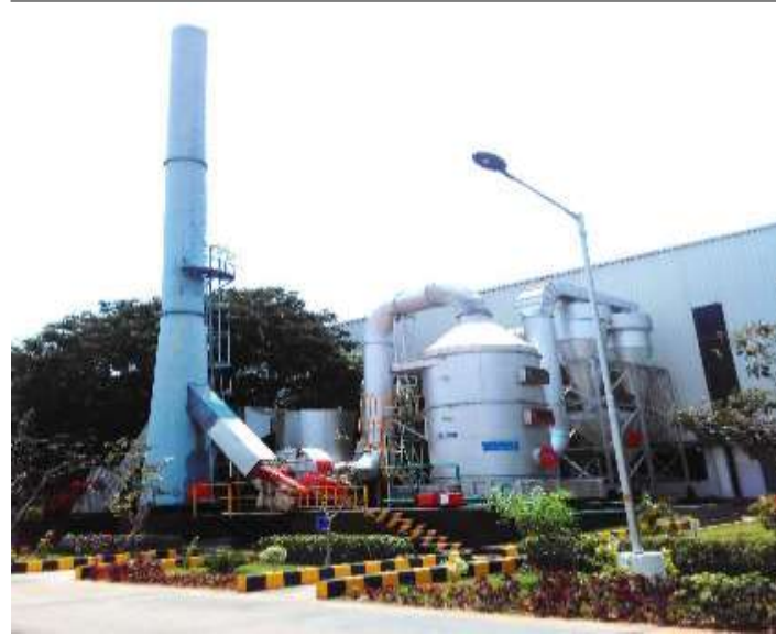
Fume extraction system with Wet Scrubbers
